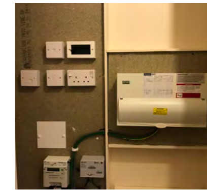
BT hub and distribution box
